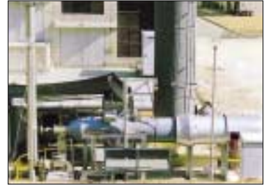
Fig 33. SCR Pilot Plant
