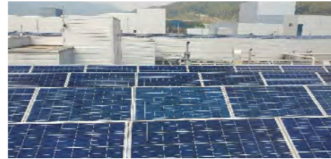
Jeungpyeong solar power plant
